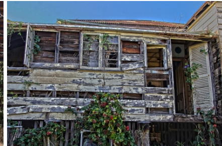
Abandoned House front Merit Doug McVicar
